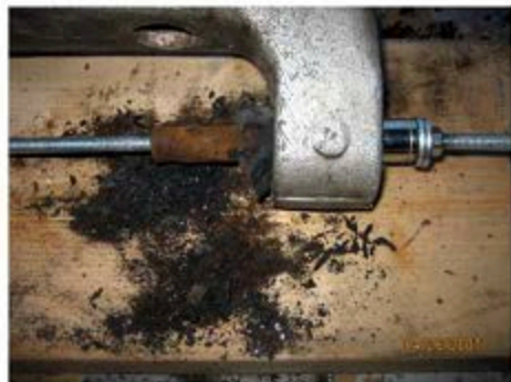
Old Bushing Almost Moved Through Hole
