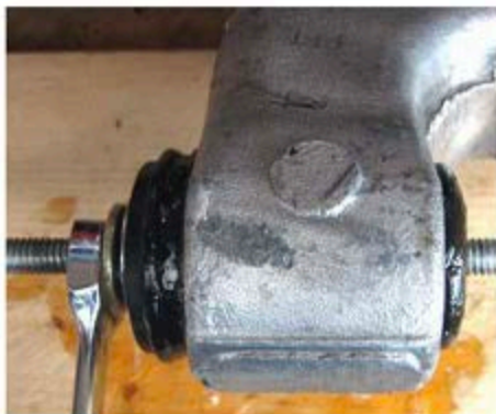
Bushing tool at initial stage of removing old rubber bushing thru T/A opening.
